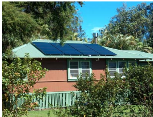
Copman Residence, Kamuela, 3.44 kW
