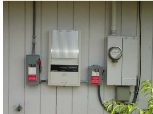
Residential 4 kW Inverter with switches
