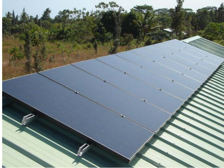
Aughe residence, HPP, 2.15 kW
